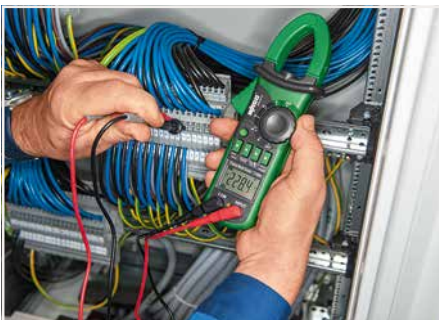
Current measurement in a switchgear cabinet
